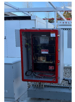
Fire Alarm Panel Located inside site
